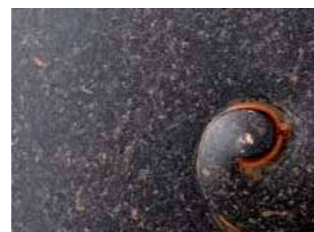
DN Rust looking
