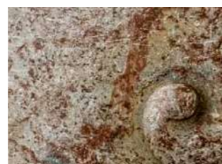
DO Watery rust
